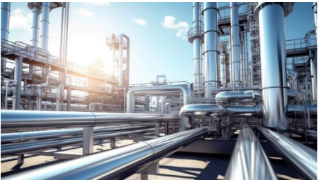
Gas supply line pipe
