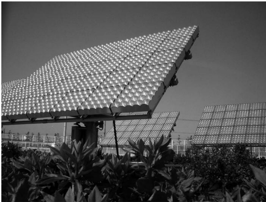
Fig.5. 30 kW concentrator photovoltaic system.
